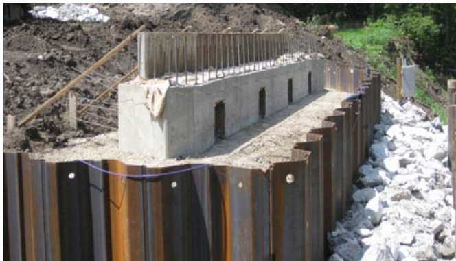
Figure 5-104. State of completion of the west abutment when zero readings were taken to determine loads and deflections for Load 1.
