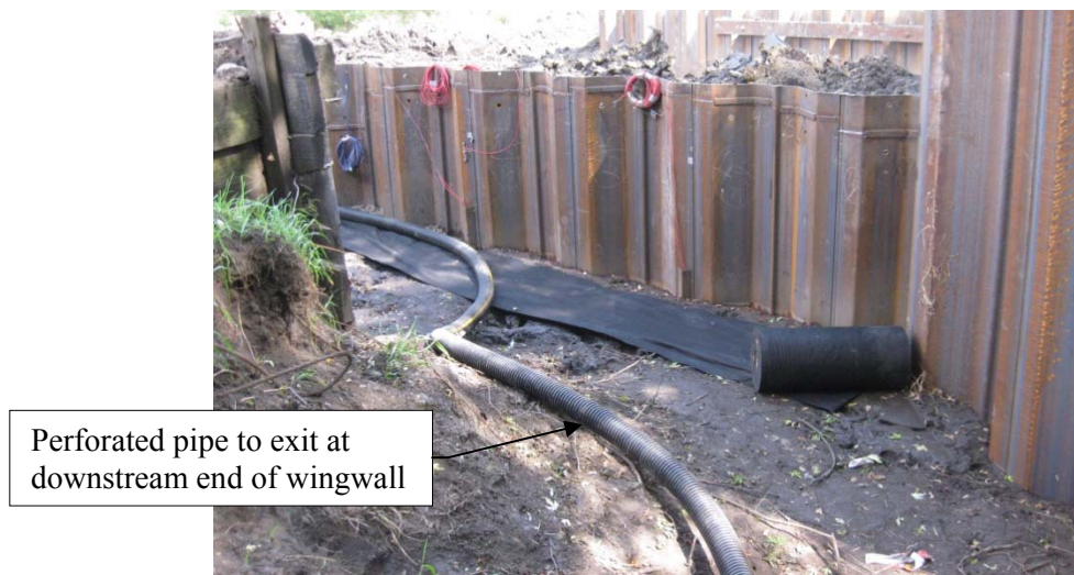
Figure 5-18. Drain tile installation on backfill side of west abutment in BHC, Iowa.
