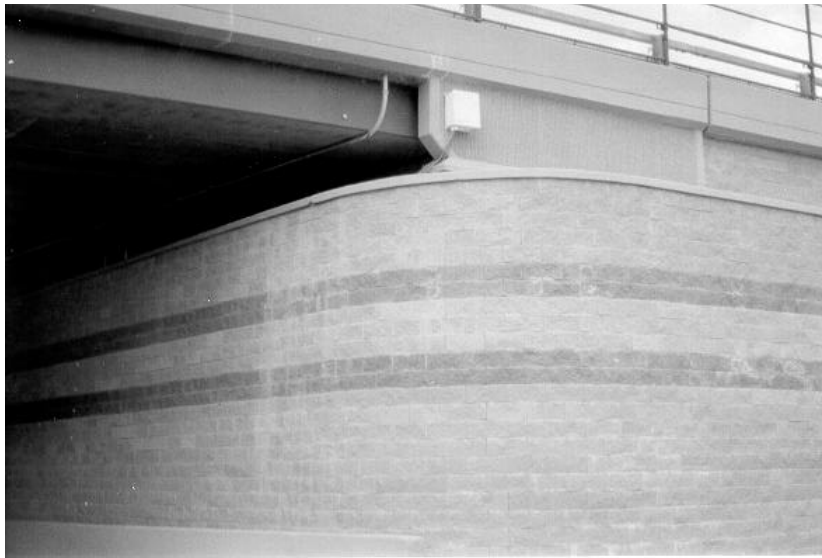
Figure 2-8. GRS abutment system for Founders/Meadows Bridge in Denver, Colorado (Abu-Hejleh et al., 2001c).
